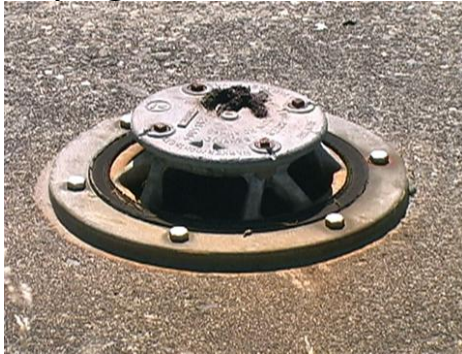
Typical Broken Light
